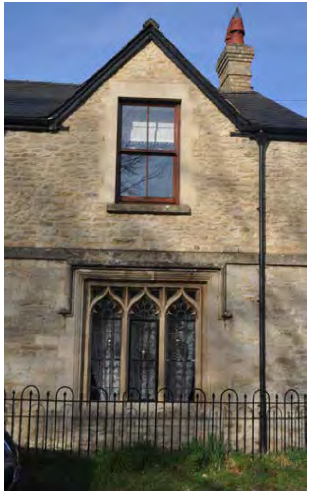
Stone mullioned window with tracery and leaded lights beneath a timber sash and case window
